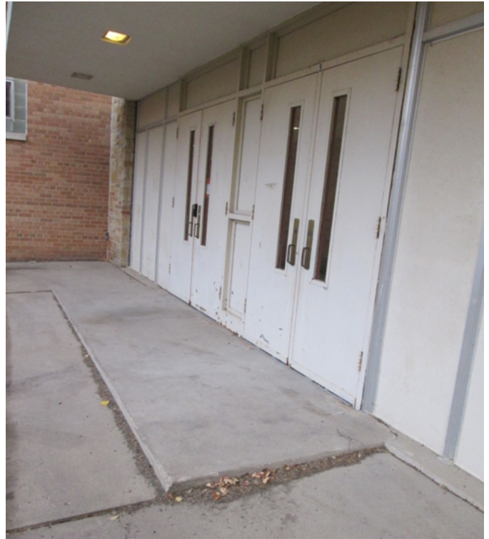
The joint sealant between the building wall and the concrete pavement is missing or deteriorated.
